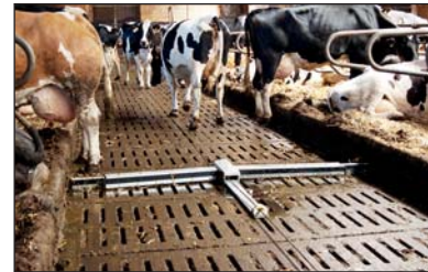
▲ 36/1 Slatted floor scraper on slatted floor
